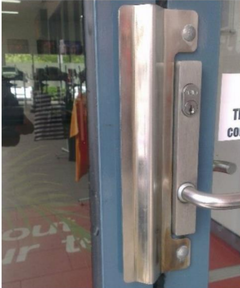
Figure 73. Large Strike Plate Cover Over Large Door Gap
