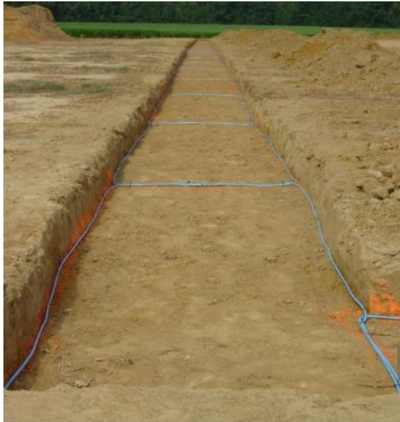
Figure 49. Cabling Hardware for UGS
