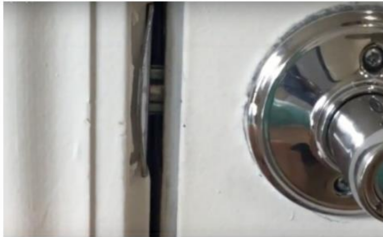
Figure 71. Shim Exploitable Door
